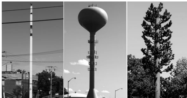
Well, They're Functional Cell transmission equipment already in place. From left: Baldwin, Lido Beach and North Hills.
